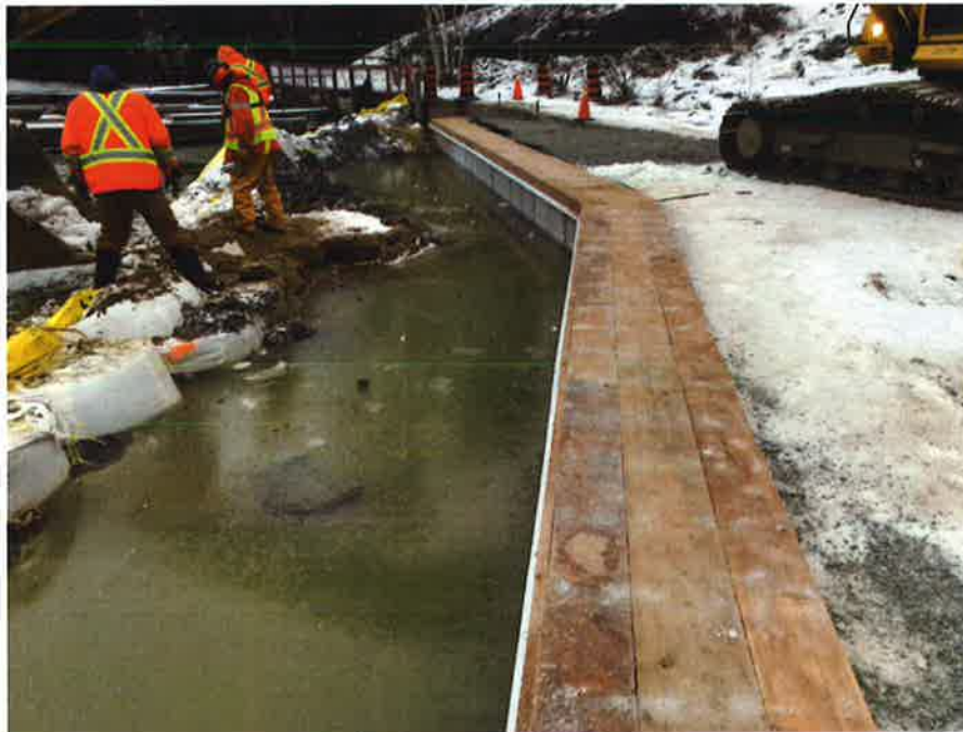
Photo 8: Progress of the Work: East wall PT wood cap, single "D" boat bumper in place.
